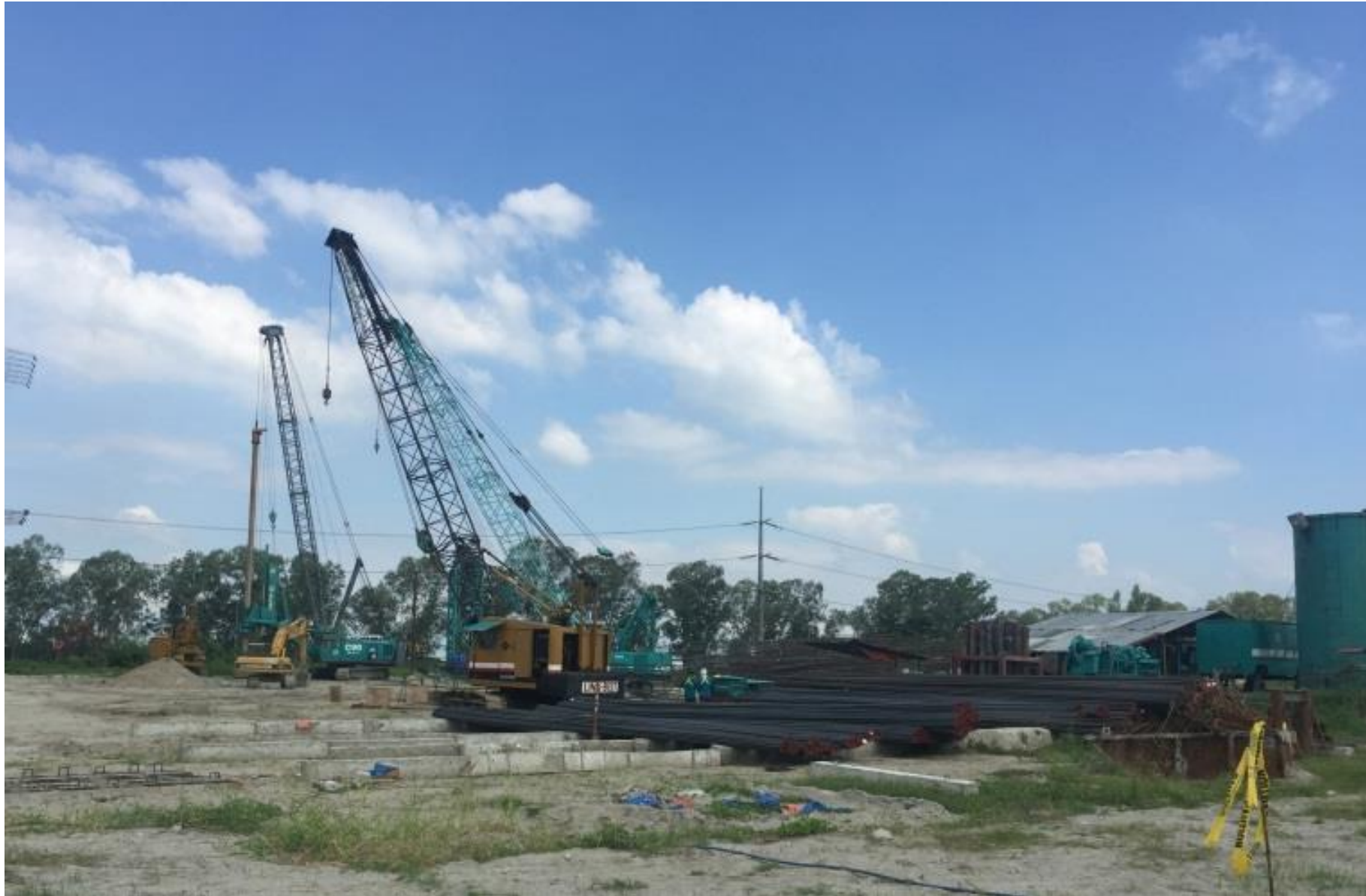
Bored piling foundation works on site and the staging area for construction
